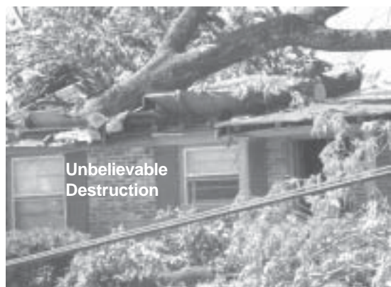
Operation Center Damaged Church Building
